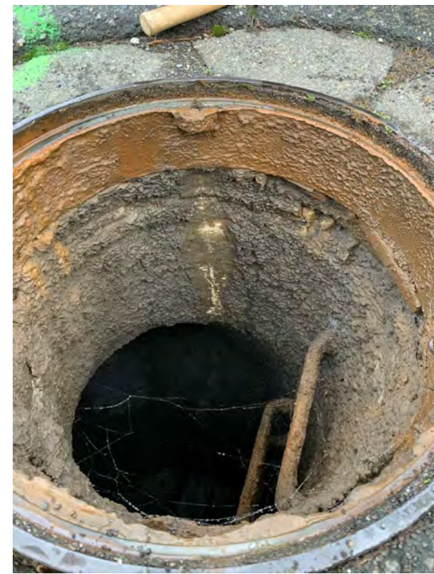
MH - 158 - ADD MAHOLE SECTION, REPLACE MANHOLE CONE, FRAME, COVER AND ADJUSTMENT RINGS AS PER DETAIL 3 SHEET 17. CONFIRM KEY-WAY PRIOR TO INSTALLATION. PROTECT SURVEY MONUMENT
