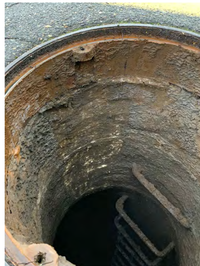
MH - 167 - ADD MAHOLE SECTION, REPLACE MANHOLE CONE, FRAME, COVER AND ADJUSTMENT RINGS AS PER DETAIL 3 SHEET 17. CONFIRM KEY-WAY PRIOR TO INSTALLATION. PROTECT SURVEY MONUMENT
